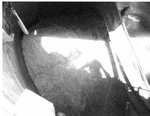
Fig. 9. Settled sediment in pond.
